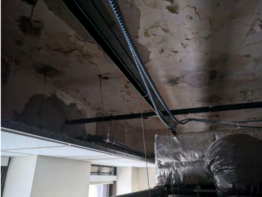
Photograph 1: Off-white paint in lead-containing paint (PC-1, 0.33%)
