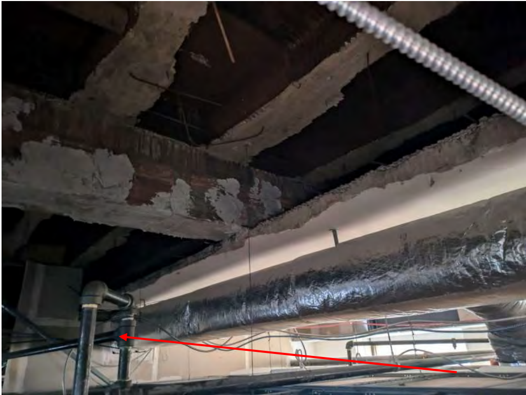
Photograph 7: Piping loop on the 14 th floor – not insulated
