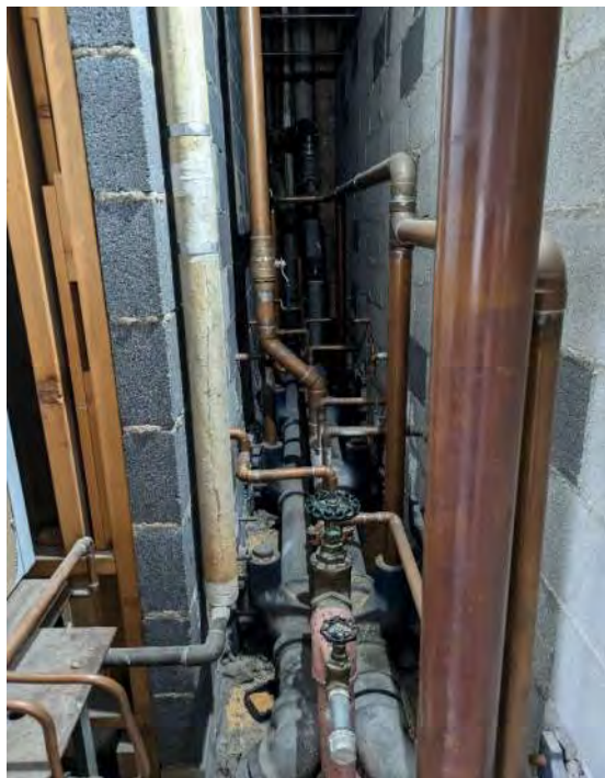
Photograph 12: 14 th floor – Bathroom, plumbing chase – asbestos-containing pipe and fitting insulation is present
