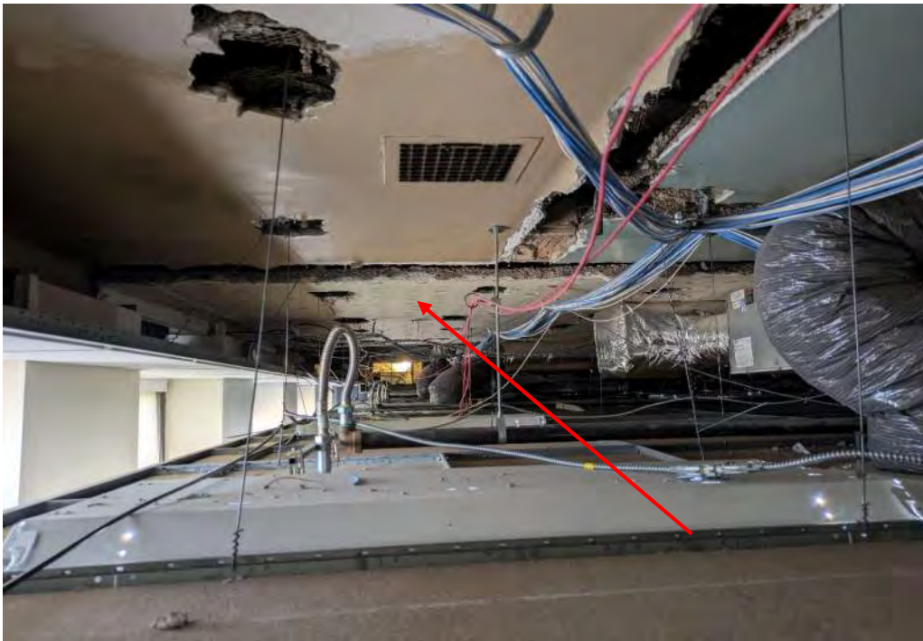
Photograph 10: View of ceiling on 14 th floor (east side of North wing, facing south) – ceiling paint is LCP / Asbestos-containing glue pods approximate location is below 1503
