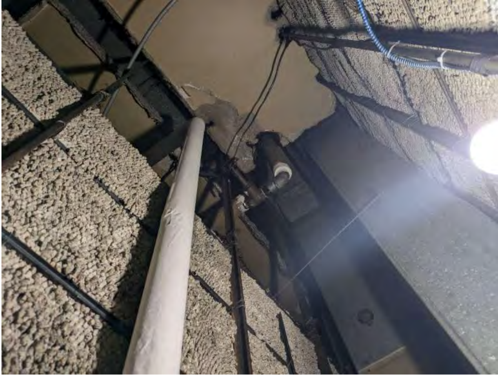
Photograph 15: ~4' length of asbestos-pipe insulation in 15 th floor bathroom plumbing chase
