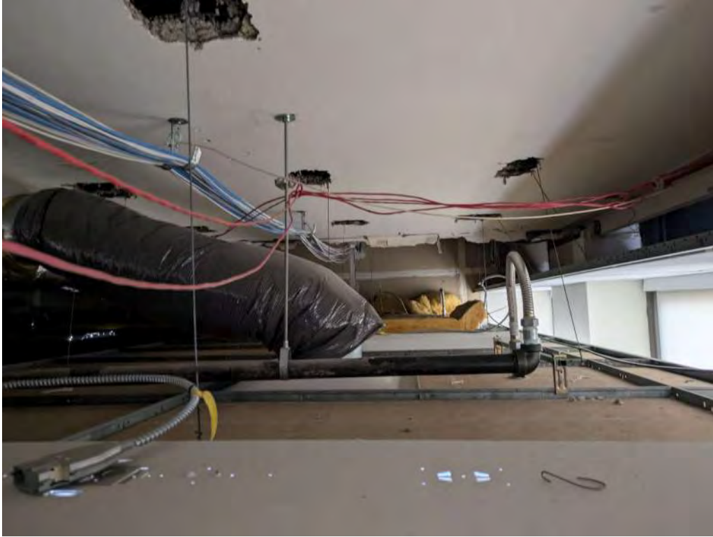
Photograph 9: View of ceiling on 14 th floor (east side of North wing, facing north) – ceiling paint is LCP
