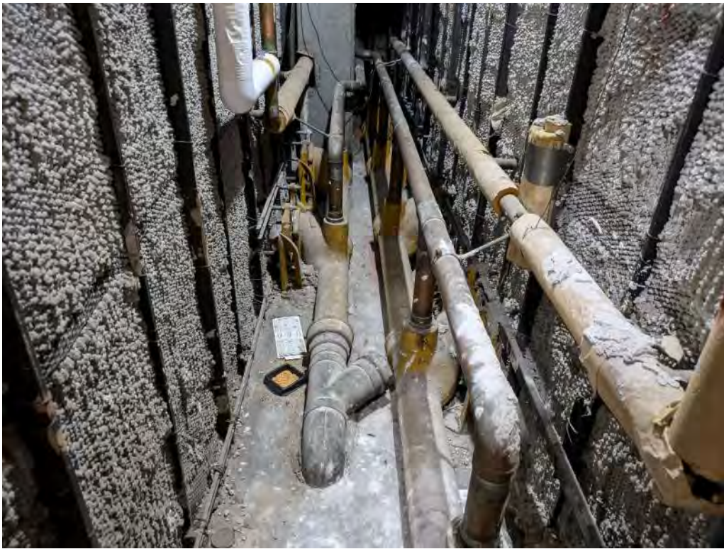
Photograph 14: White debris on pipes and floor (HA #8) – non-ACM
