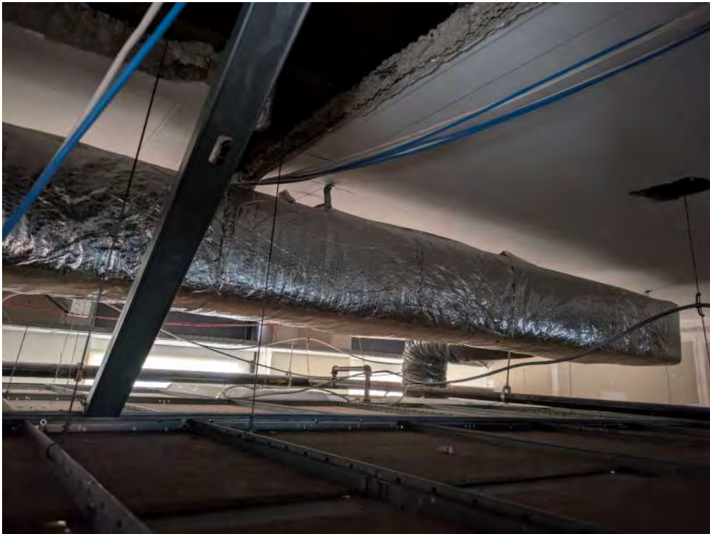
Photograph 8: View of ceiling on 14 th floor (west side of North wing) – ceiling paint is LCP
