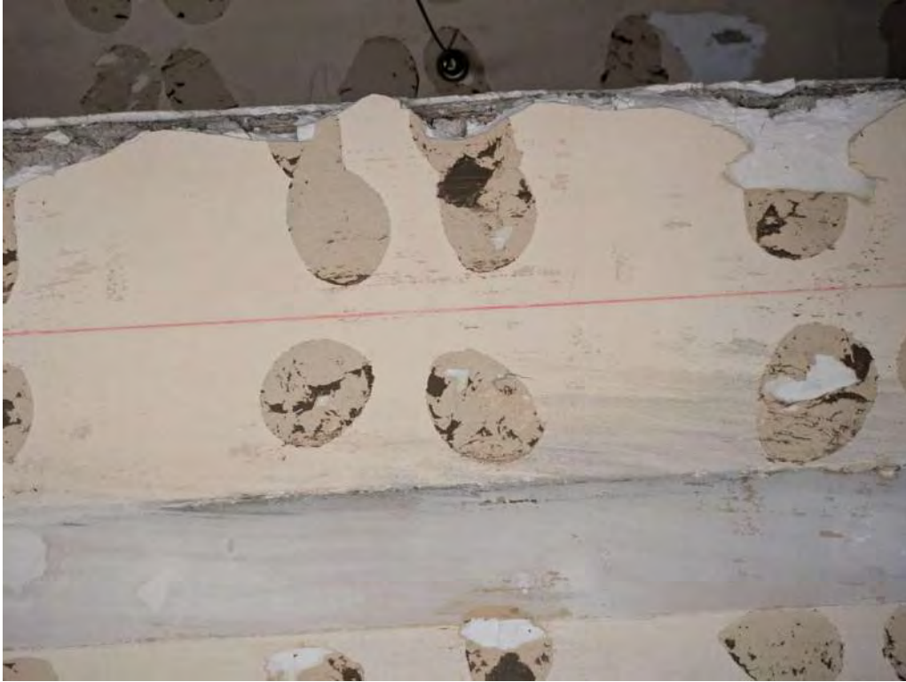
Photograph 3: Remnants of brown glue pods (HA #2) – contain asbestos
